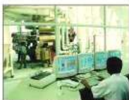
Fully Computerized Control System (From raw material receiving to finished products storage)
